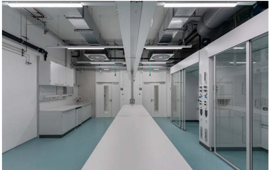
Chemical lab with walkable fume hood
